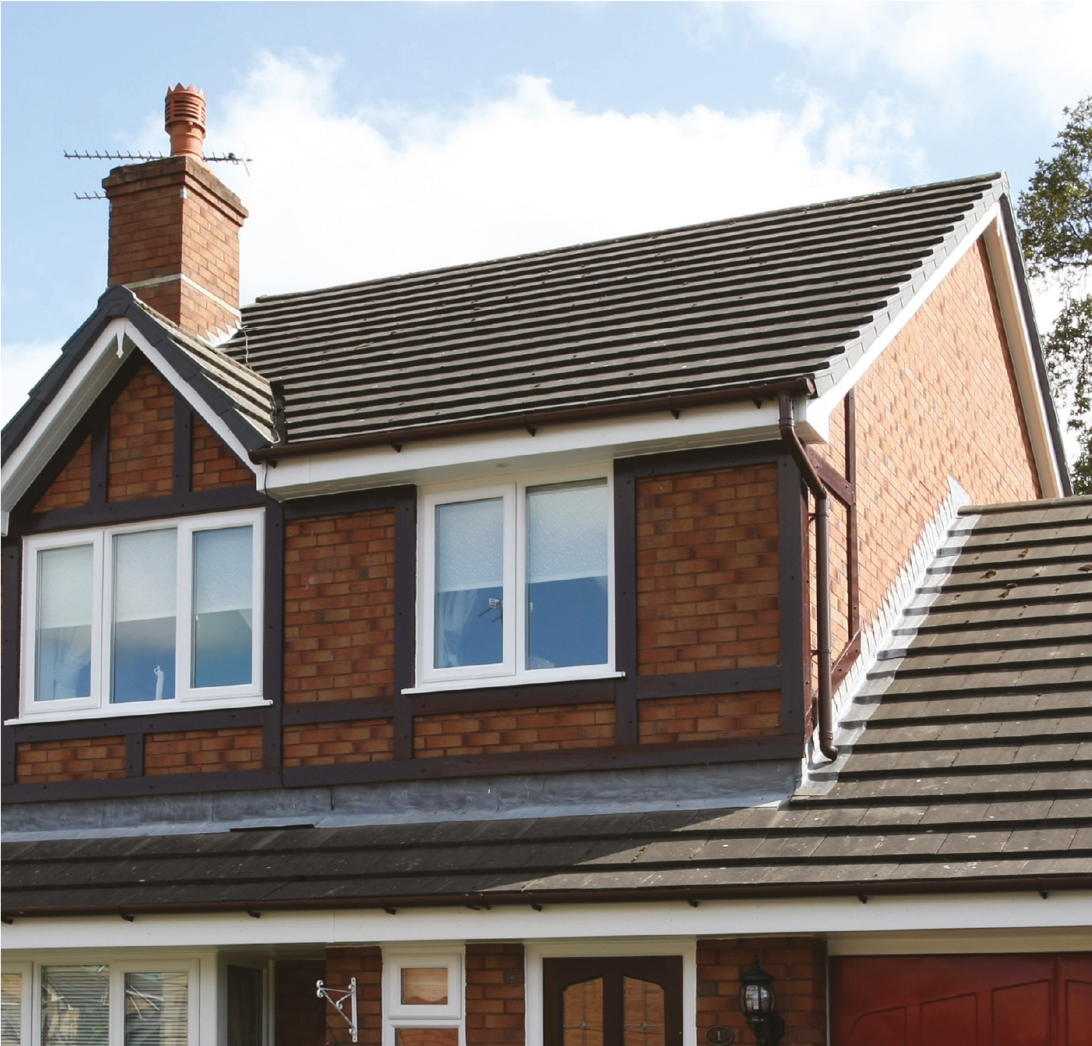
Detached property with White square fascia boards and grooved soffit boards, finished with half-round guttering in Brown.
